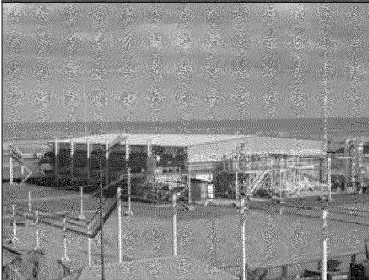
New Gas Compression Plant at Borankol
