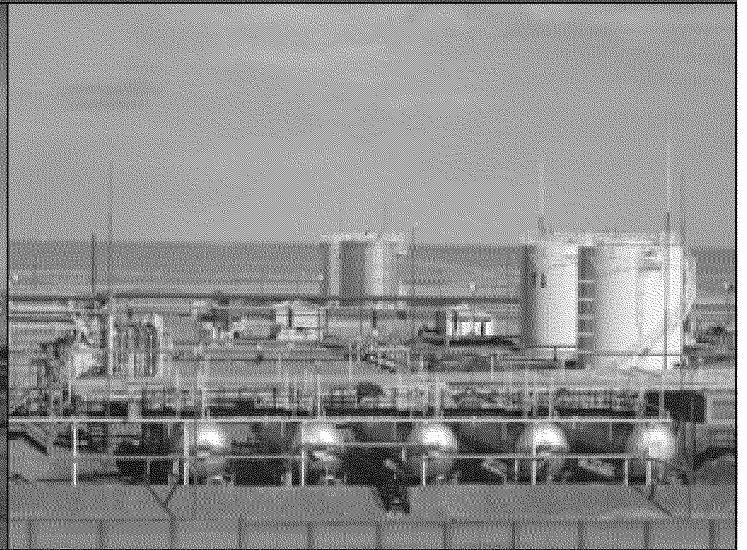
Condensate Storage at Tolkyn Gas Plant
